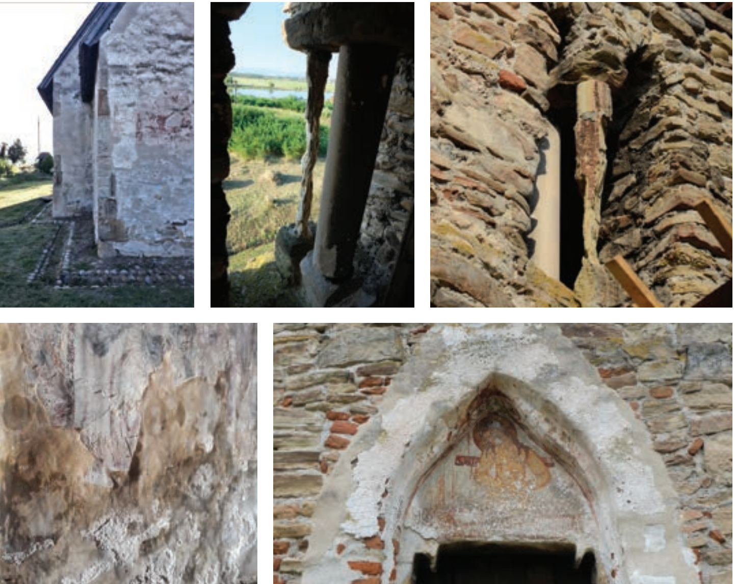
▲ Fig. 9-13. Degradations of the medieval exterior paintings of the Strei church, of the old colonnettes in the tower, and of the western portal (2017).
