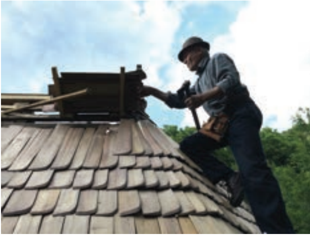
▲ Fig. 3. Master Nicolae Toader working at the Vălari church, 2018. ▼ Fig. 4a and b. The medieval church in Gârbova de Sus before and after the roof installation.
